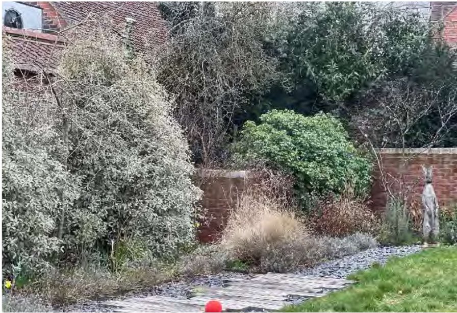
View of application site from rear garden to corner of garden showing retaining wall (looking north-west)
